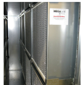
MEGAcel® I filters installed in Cancer Treatment Centers of America.®
