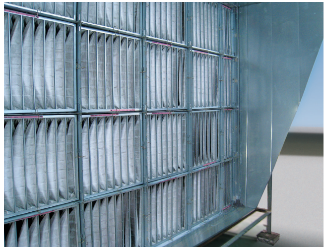
VariCel® M-Pak filters installed in recirculation units (top) and DriPak® 2000 filters installed in fresh air intakes (bottom) at 777 Main Street, Fort Worth, TX.
