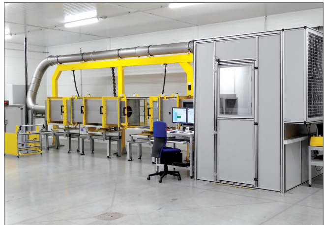
AAF ISO 16890 Testing Facility
